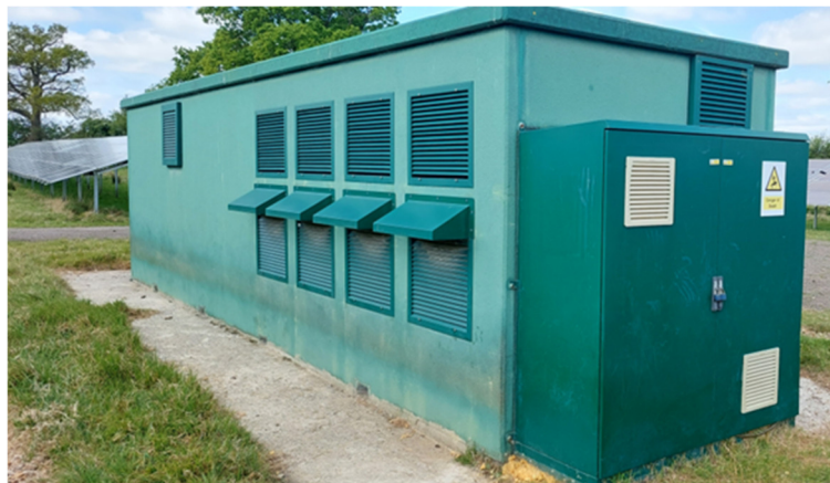
Plate 2: Typical Inverter Station
